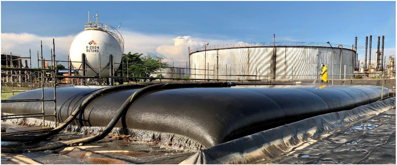
Figure 7 – Before and After Separator Chamber SE3090
