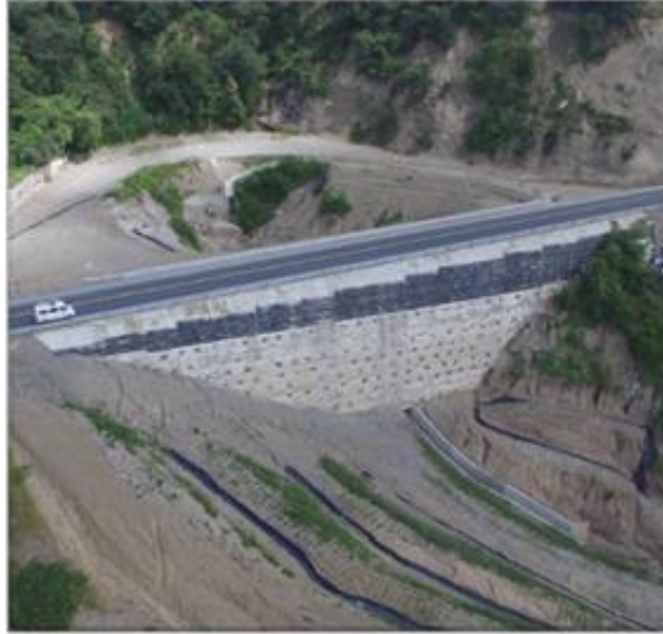
Figure 7 State of the Wall before placing the facade in erosion control mantle
