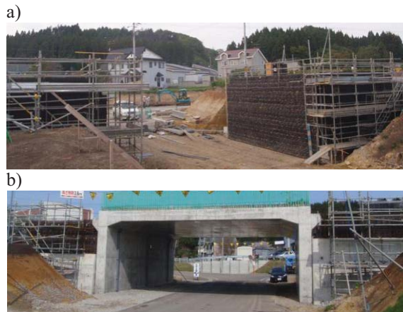
Fig. 15 First prototype GRS integral bridge (11.7 m-wide) for a new high-speed train line, Kikonai: a) general structure (by the courtesy of Japan Railway Construction, Transport and Technology Agency); b) during construction (Oct. 2011); and c) nearly completed (June 2012).
