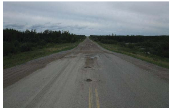
Fig. 4 Excessive settlement and lateral movement of a road on degraded permafrost along Provincial Road 391 in Manitoba.
