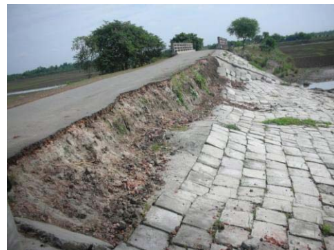
Fig. 1 Slope failure in an earth fill embankment
