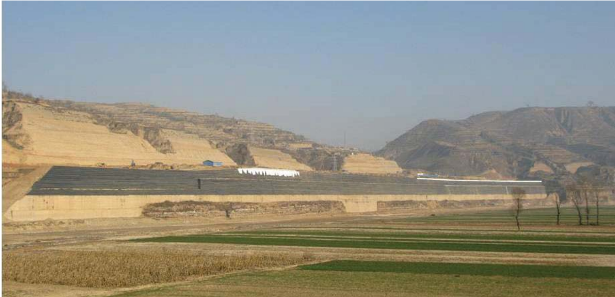
Fig. 13 Oblique frontal view of the substantially completed geotextile reinforced soil wall at Hetaoyu
