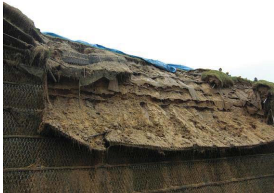
Fig. 1a Reinforced soil wall deformation
