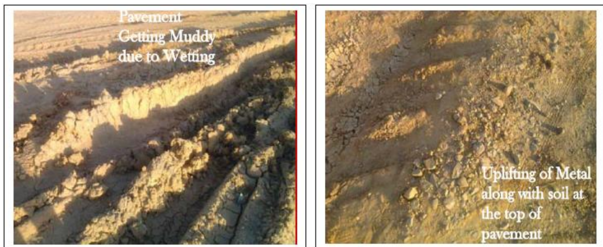
Figure 2. Photographs illustrating deformed pavement condition at site.
