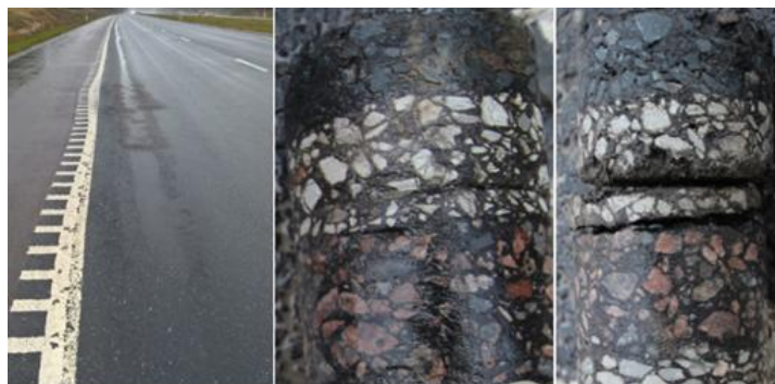
Figure 3. Bonding problems between glass fiber grid and pavement was noticed.
