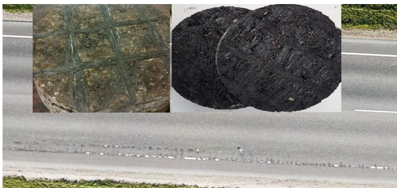
Figure 5. Left core sample was taken from damaged (shown below) and right undamaged section
