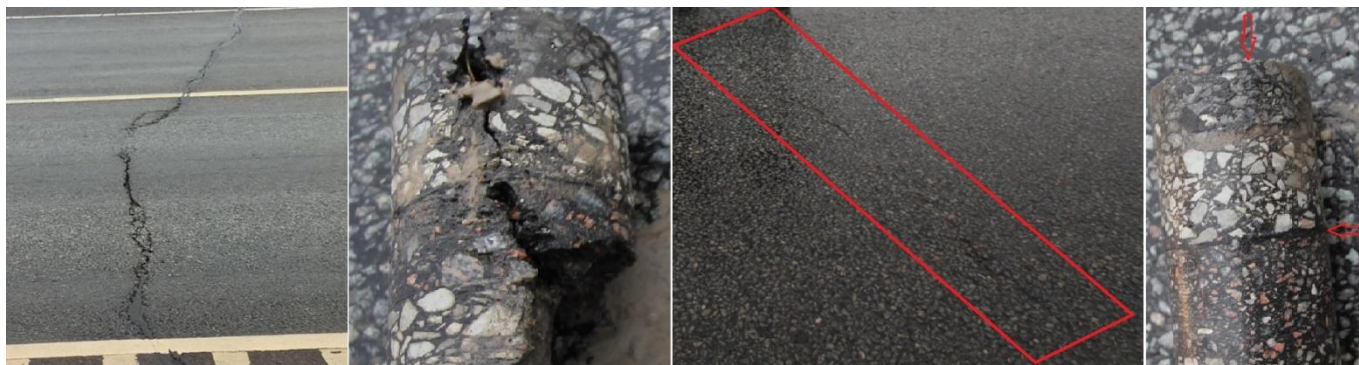
Figure 2. Transverse cracks in different stages – one is repaired and has appeared to the same location as it used to be and second one is new, unrepaired. In both cases paving fabric was used.
