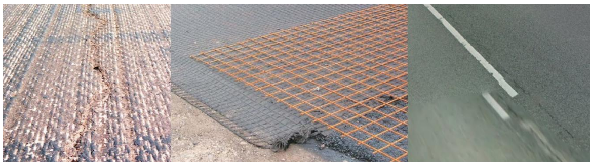
Figure 1. Longitudinal frost heave crack before rehabilitation, installation of PET and steel grid, longitudinal frost heave crack 7 years after roadworks [photo courtesy: Enno Vahter]
