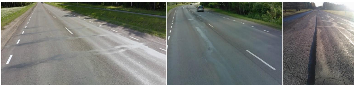
Figure 4. Defects found in third test section before rehabilitation works.
