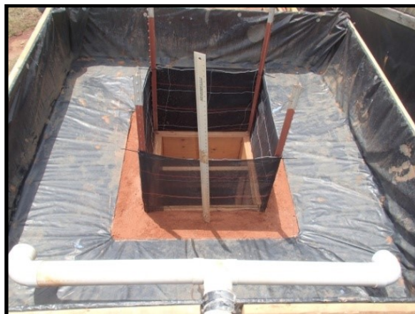
Figure 12. Close-up of a Typical Installation
