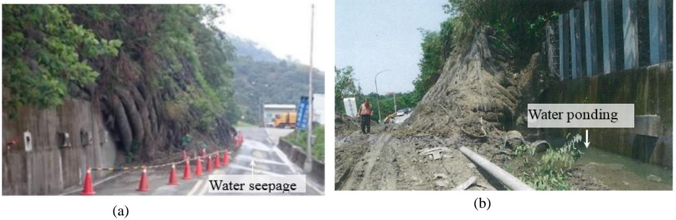
Figure 4. Slope failure: (a) slope toe with water seeping out from backfill; (b) another view at the slope toe with water ponding (from Taiwan Professional Geotechnical Engineers Association report, 2014)
