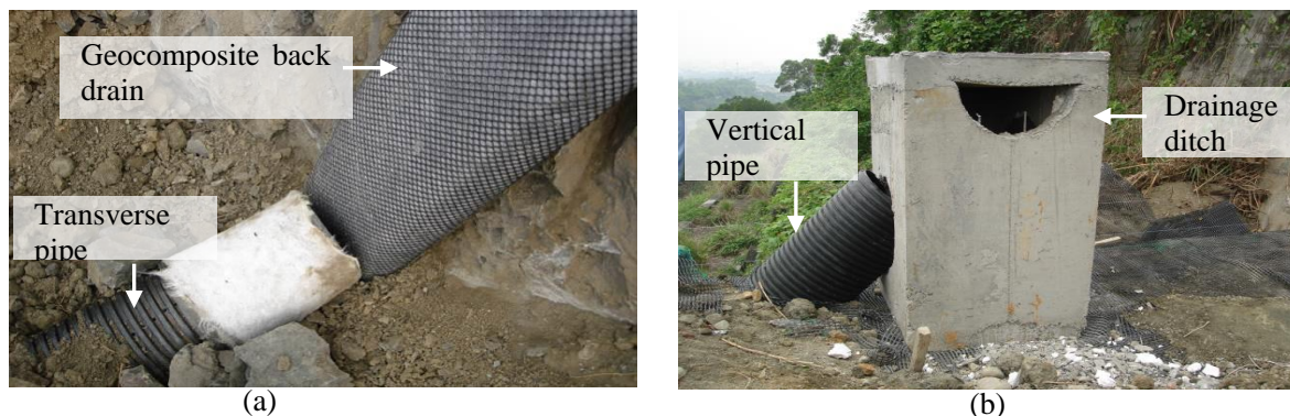
Figure 2. Drainage installations: (a) connection joint between back drain and transverse pipe; (b) connection joint between drainage ditch and vertical pipe (from Taiwan Professional Geotechnical Engineers Association report, 2014)
