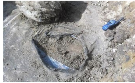
Figure 2 Hole caused by oversized aggregates
