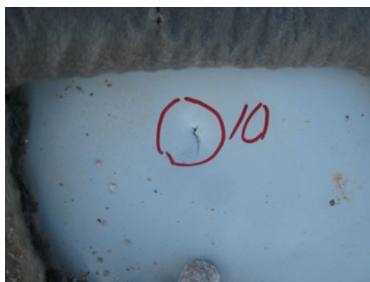
Figure 11 Example of leak detected
