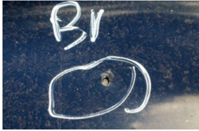
Figure 1 Defect caused by welding process
