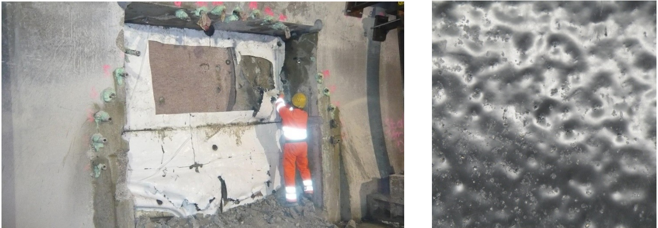
Figure 2. GBR-P samples taken from an old road tunnel at the location of a new cross passage (picture: left: ABD Südbayern, right: BAST).
