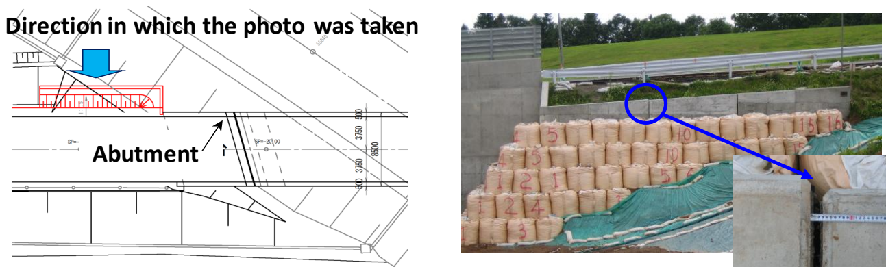
Figure 3. The deformed reinforced soil wall and the deformation control work.
