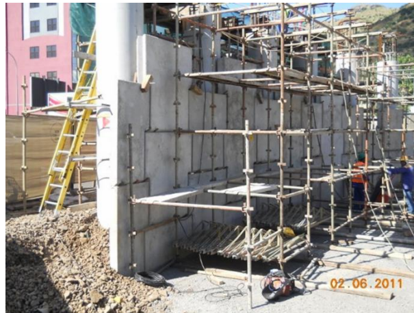
Figure 1. MSEW with bridge piers – issues during construction
