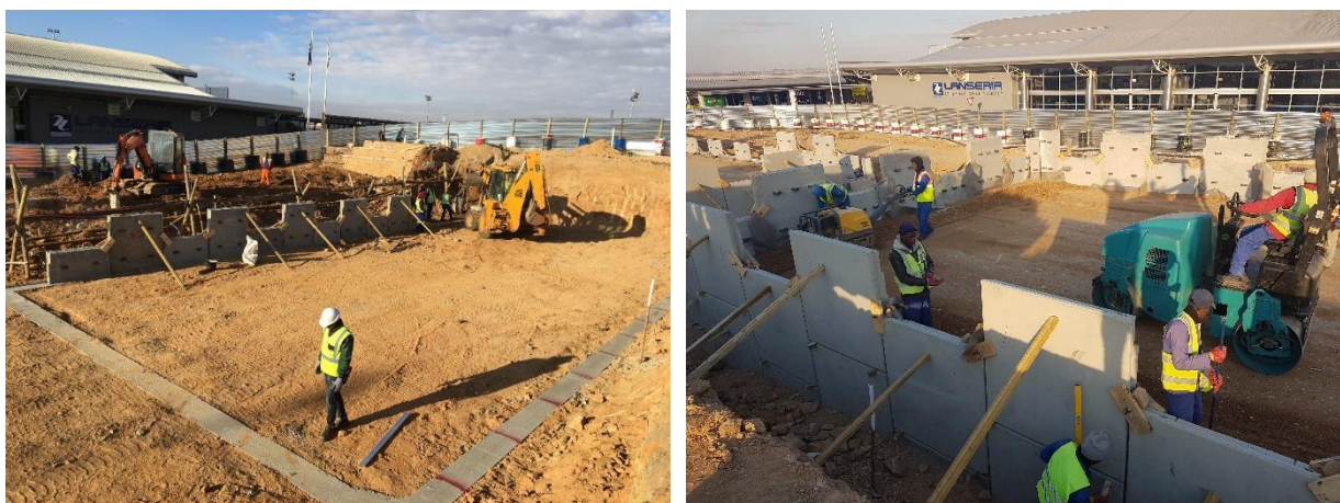
Figure 8, 9. Foundation and levelling pad with first row of panels / Different compaction techniques used in the backfill
