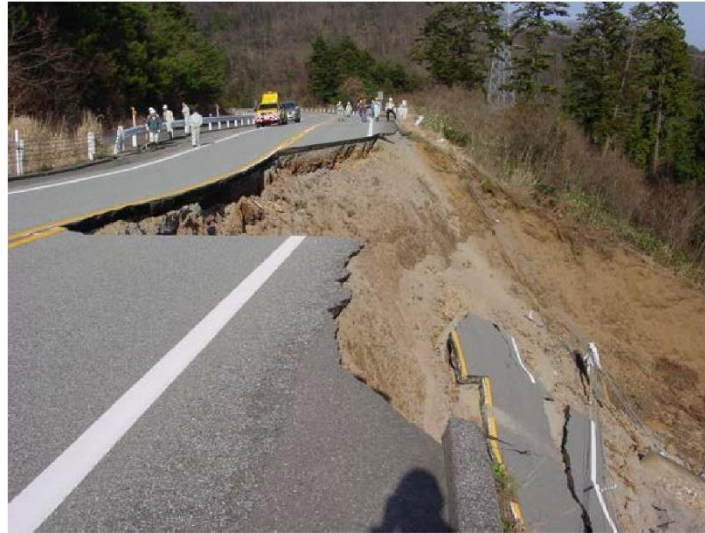
Photo 1. Damage of road embankment during 2007 Noto-peninsula earthquake.
