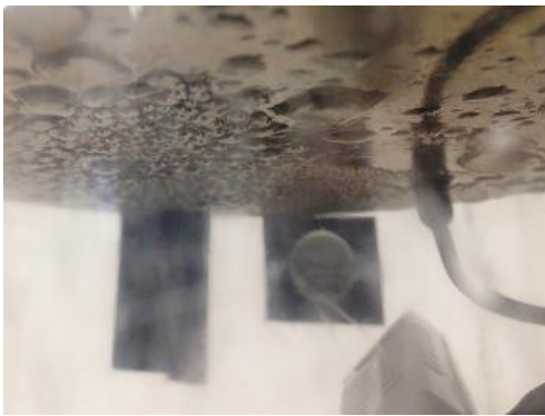
Figure 6. Image of condensation
