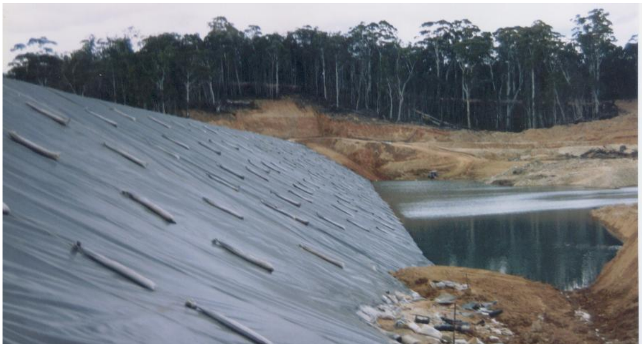
Figure 2 A lined upstream face of an embankment of a tailings dam with sand filled ballast tubes suspended on the slope
