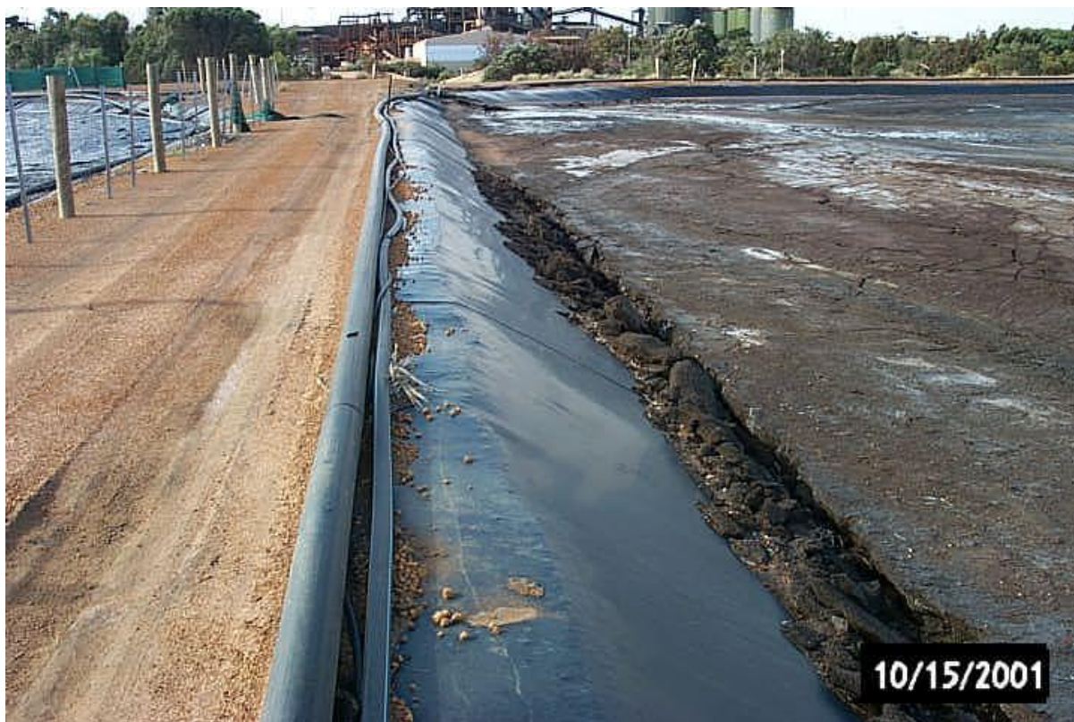
Figure 3 A lined tailings dam where the tailings have dried and settled leading to down-drag on the liner
