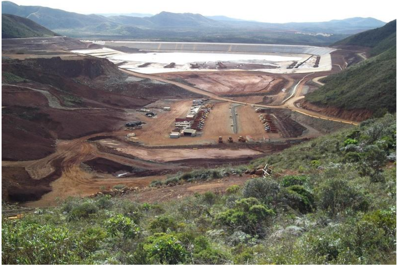
Figure 1 A large tailings dam in the tropics with a geomembrane liner where many issues associated with wind and stormwater were addressed.
