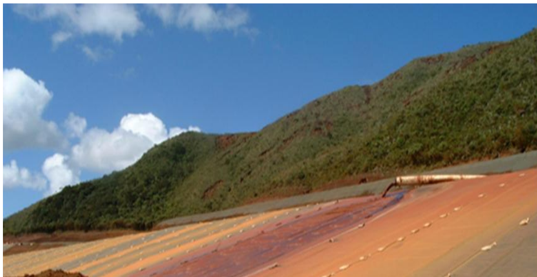
Figure 6. A pipe discharging hot slurry directly on to a liner
