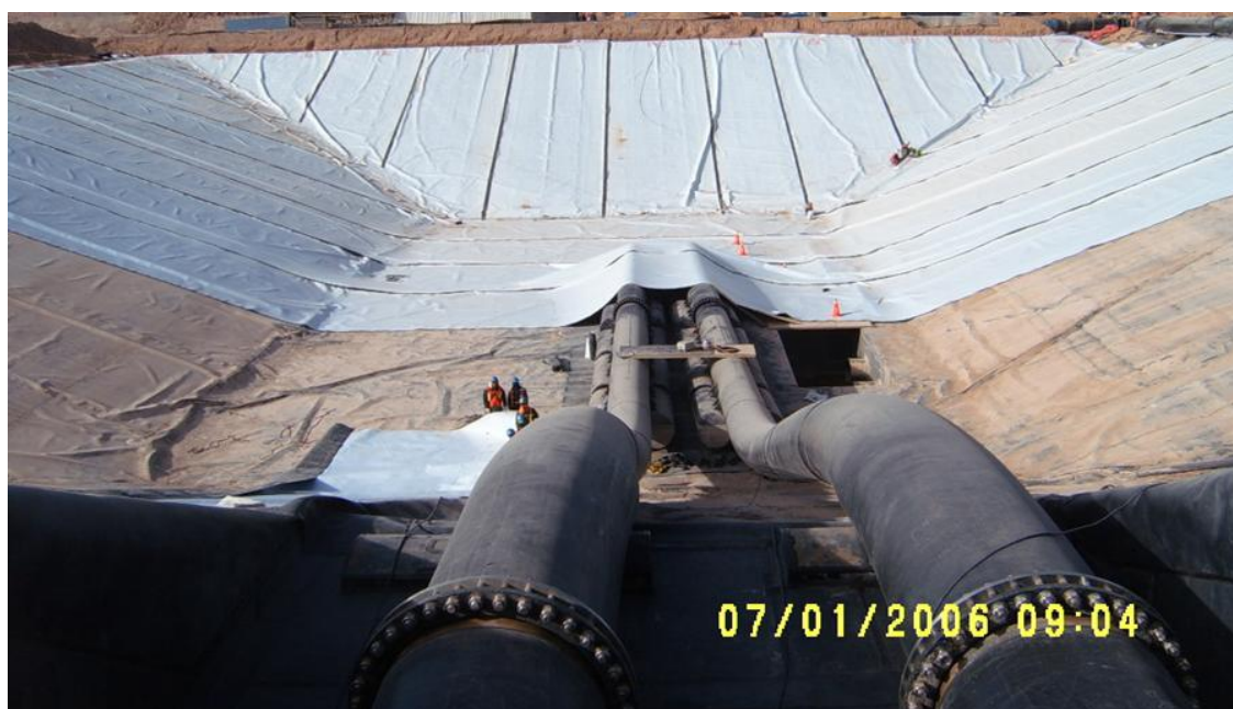
Figure 7. HDPE pipes with floats so that discharge is away from liner. These pipes are shown entering the facility beneath a cover, and the floating exits of the pipes are well above the liner.
