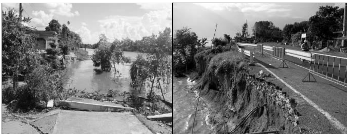
Figure 3: Failed section of roads in the Mekong Delta
