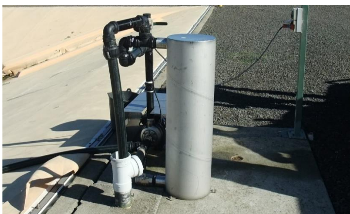
Figure 1. An off-cover pump arrangement. The pump discharges to the header tank which overflows to a drain.
