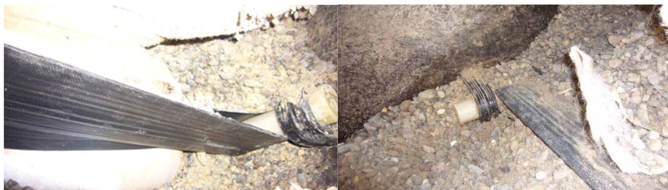
Figure 6. Condition of connections between reinforcement and facing panel
