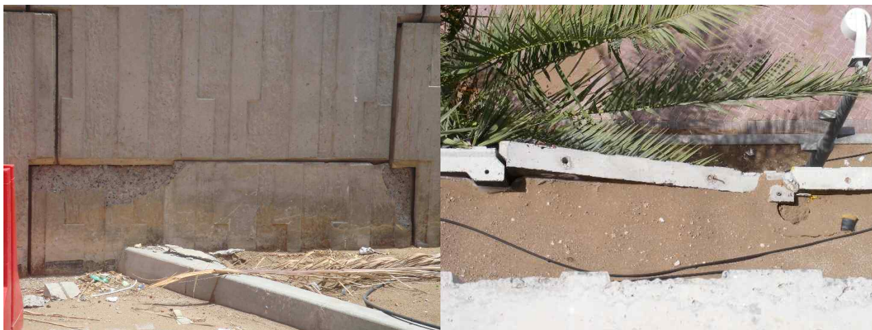
Figure 2. a) Damage near the bottom of the wall; b) Panel movement observed from top
