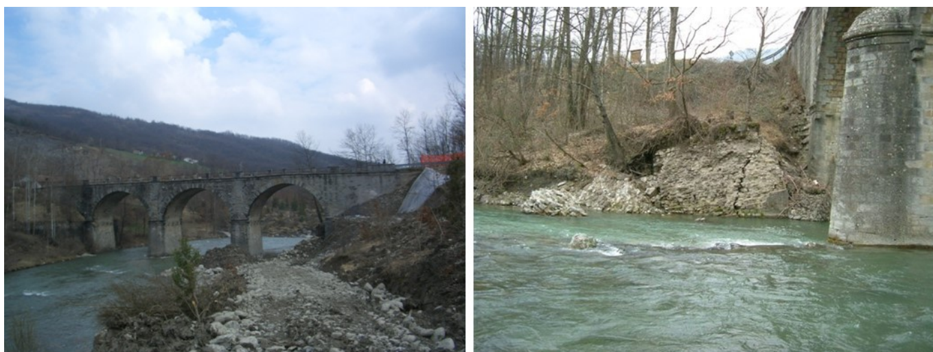
Figure 9. The Ponte Prugneto historical arch bridge and the failure of the upstream wing wall
