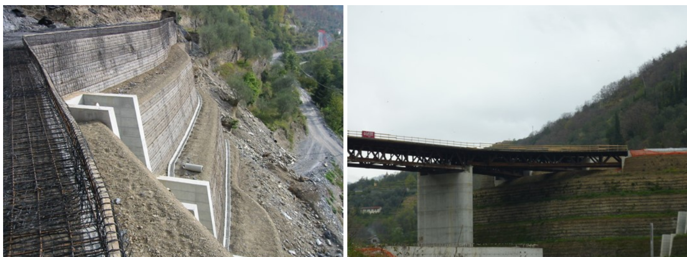
Figure 4. The wall under construction, showing the concrete channel for the Rio Teco creek, and the bridge abutments on top of the wall
