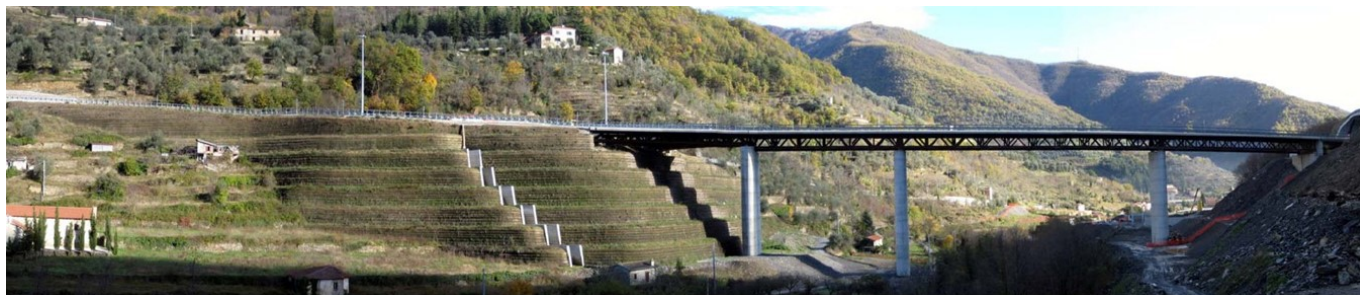
Figure 1. View of the reinforced wall of the Northern roundabout with the bridge abutments on top
