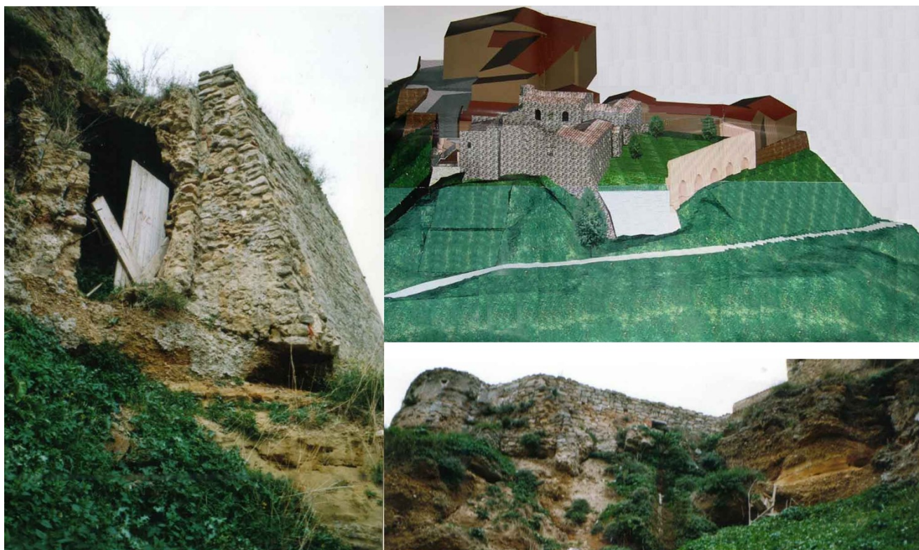
Figure 14. 3D reconstruction of the Church – Monastery complex and pictures showing the highly degraded state of the slopes with the formation of caves just below the foundations
