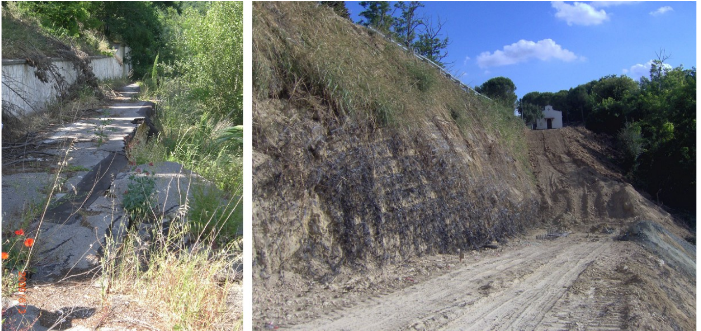
Figure 17. Failure of the road in Farfa and subsequent excavation for the reinforced soil structure
