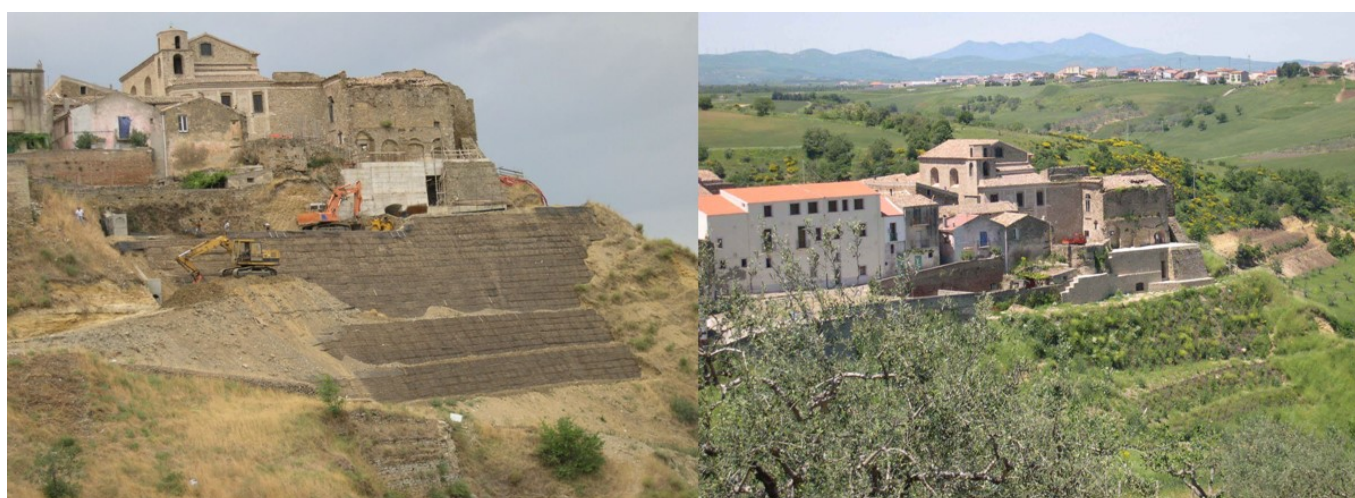
Figure 16. The reinforced soil wall during construction and the final vegetated reinforced soil structure
