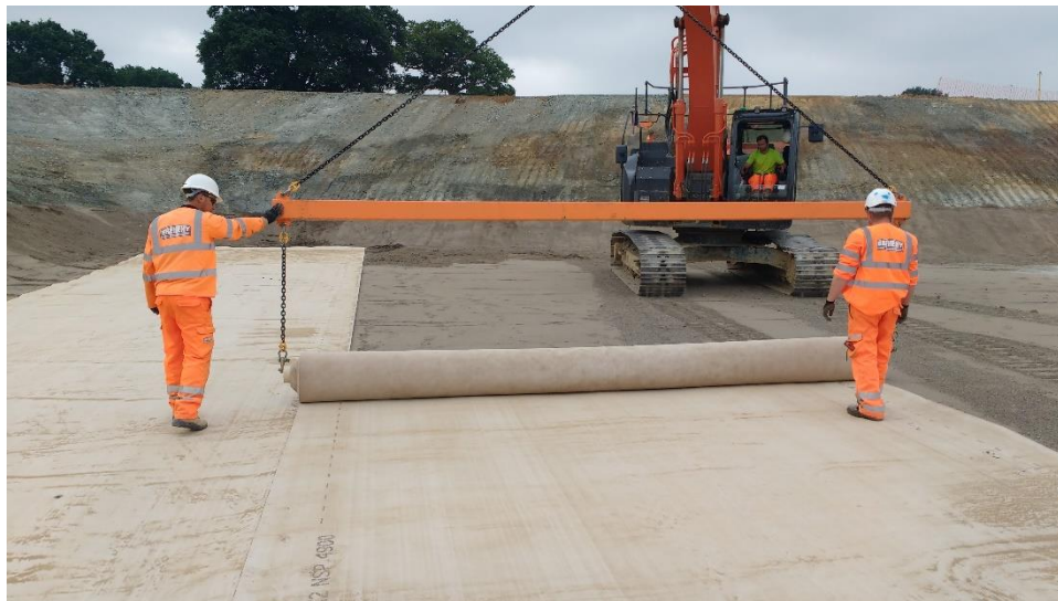
Figure 5. Coated GCL being installed as the essential seal in each water storage basin
