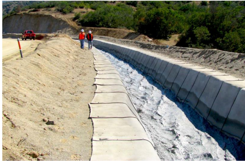
Figure 3. Use of a GCCM to line a tailings ditch carrying liquid made up of up to 60% solids
