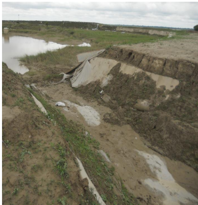
Figure 7. Breached portion of the dyke
