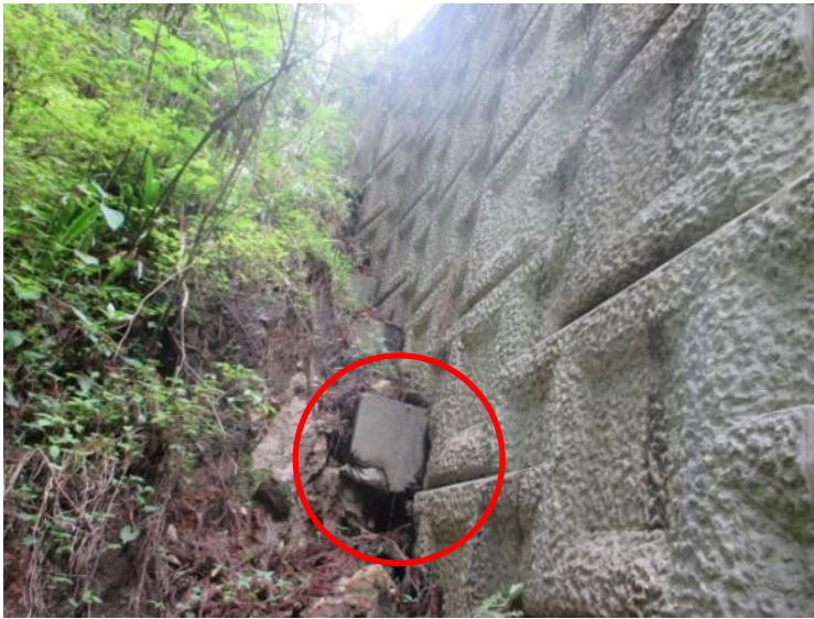
Figure 5 Scouring under foundation
