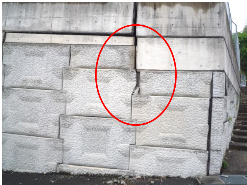
Figure 2. Gap separating two panels
