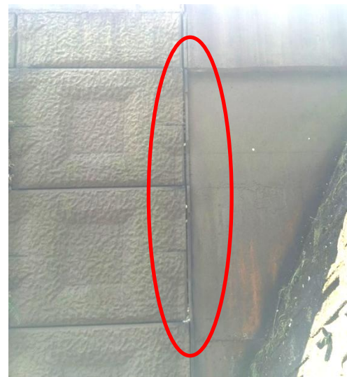
Figure 6. Elongation between panels and adjacent structure
