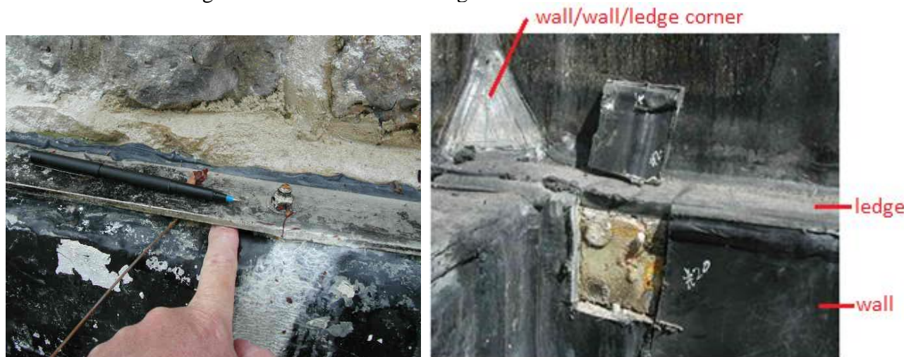
Figure 16. Unsatisfactory batten bar support (left) and CPL welds (right).
