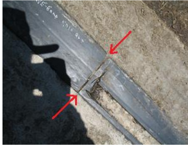
Figure 11. Joint (arrowed) should be welded
