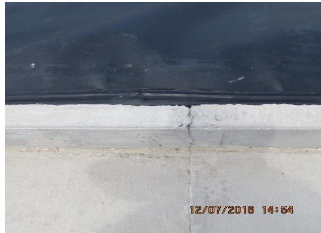
Figure 13. Crack in concrete under the batten strip.
