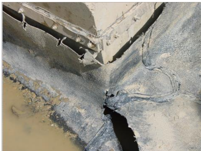
Figure 14. Geomembrane not supported in corner.
