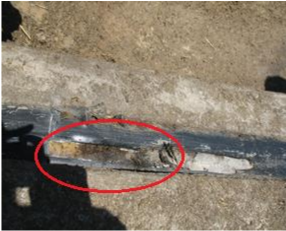
Figure 10. Rough concrete surface with air space (circled) has allowed leakage. Half of top of embedment strip removed.
