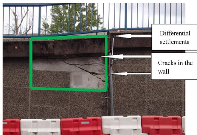
Figure 3. damages on the wall.
