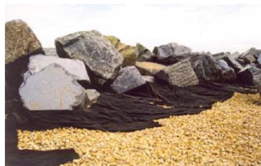
Figure 4: Mismatch of permeabilites of geotextile and underlying layer
