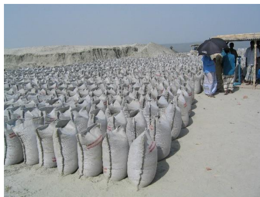
Figure 25: hand filled bags ready for loading on to a barge for dumping
