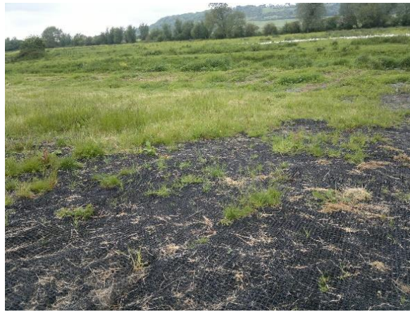
Figure 21: Worst area where only surface topsoil lost and synthetic root structure maintained a hydraulic shape to prevent further erosion whilst in grassed areas as it reinforced the existing roots
