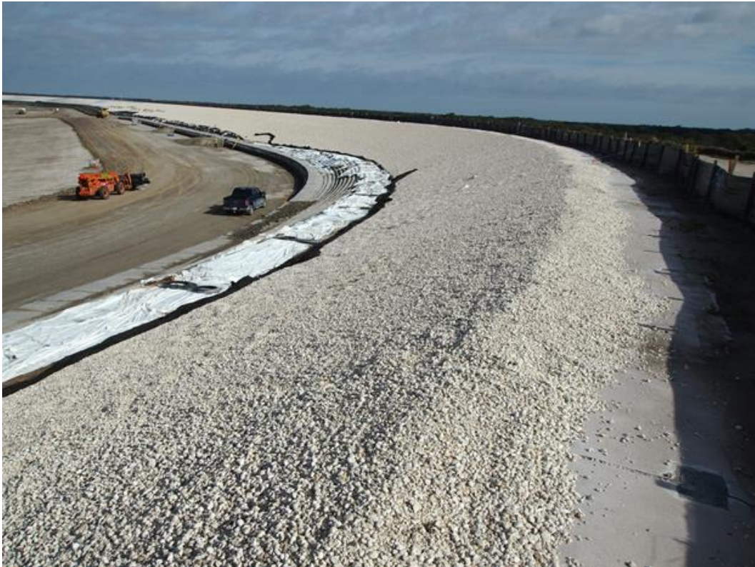
Figure 6: The soil-cement finishing over the sealing system in the Bill Young Reservoir project
