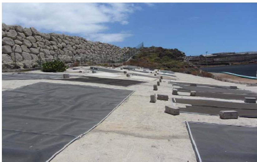
Figure 1. Partial view of the experimental field of synthetic geomembranes in the reservoir of El Saltadero
