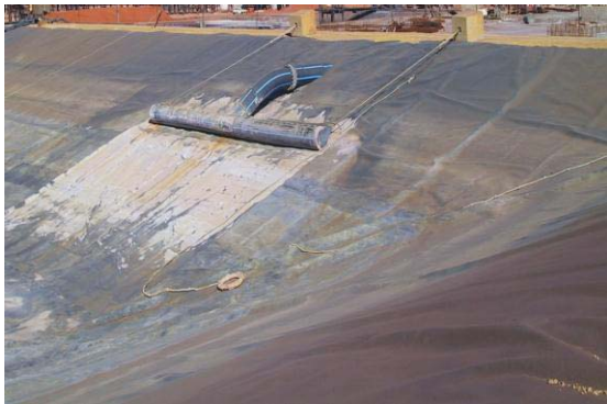
Fig. 3 An unusual inlet pipe and distribution arrangement
