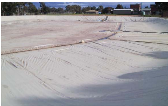
Fig. 32 A floating membrane cover to a water storage facility
