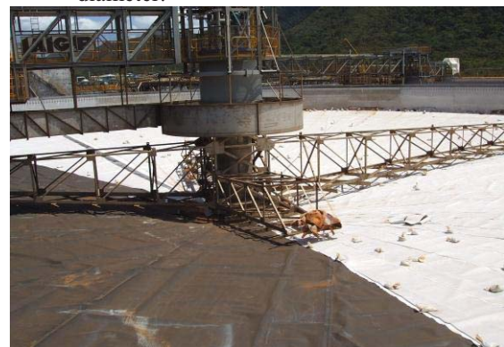
Fig. 5 A large (70 m diameter) CCD thickener with a primary liner being installed over a geocomposite. The rake clearance is less than 200 mm to be effective.
