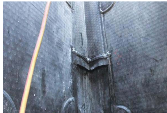
Fig. 12 Corner cover strips subjected to external water pressure when tank is empty
