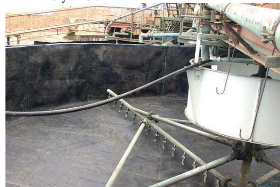
Fig. 4 A relatively small thickener with rotating arms and racks to draw the slurry towards the central outlet. This one is about 10 m in diameter.
