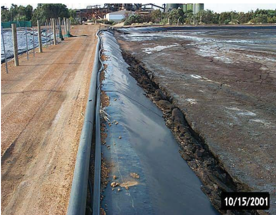
Fig. 8 A tailings pond with the tailings drying at the perimeter more than the centre which leaves the tailings tending to slide down the face of the liner imposing significant downdrag stresses.
