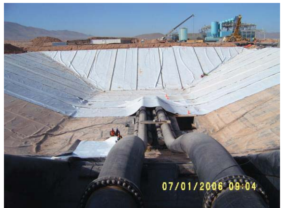
Fig. 2 A floating cover for a copper mine PLS pond being installed over two 900 mm diameter inlet HDPE pipes
