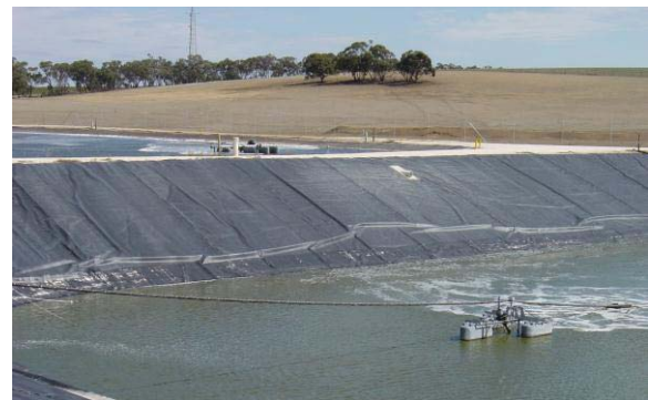
Fig. 26 HDPE lined lagoon with floating surface aerators
