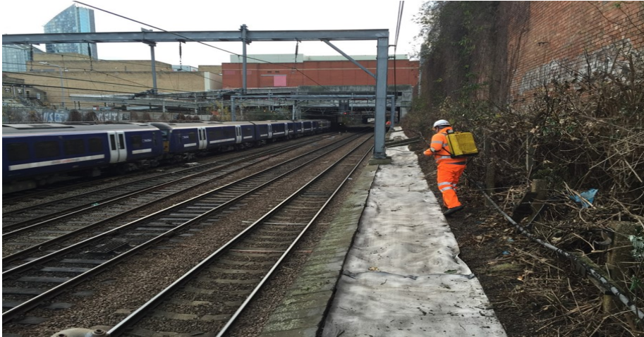
Figure 3. GCCM used for weed suppression, mobilisation of shotcrete equipment was not possible without major shut down of train lines
