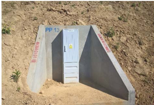
Photo 1. An example of the measuring point - view of cabinet measurement in concrete enclosure
