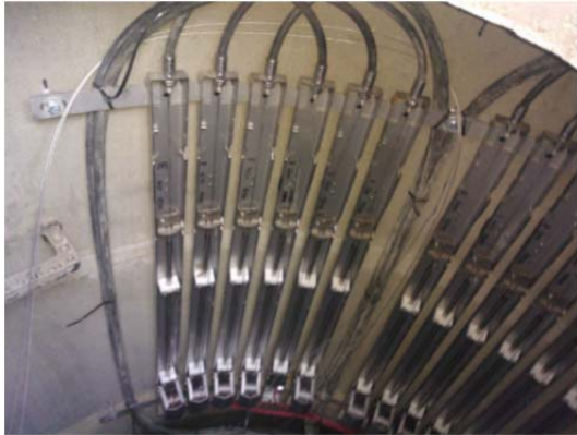
Photo 3. The view of the sensors which monitoring the vertical displacement of soil
