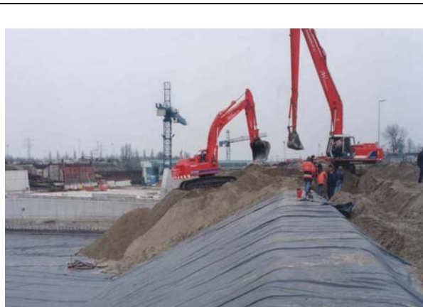
Figure 15. Risk to instability soil backfill and severe damage geomembrane, using a wrong backfill sequence at the geomembrane structure [Ref. Dutch directorate for public Works and Water Management]
