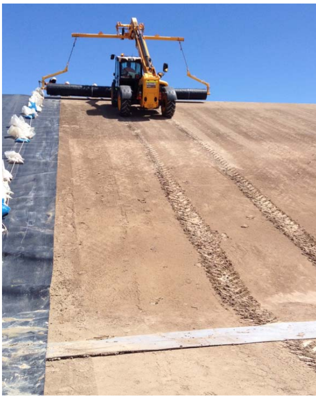
Figure 11. Unacceptable damage to sub grade and improper working method by construction equipment [Scheirs]
