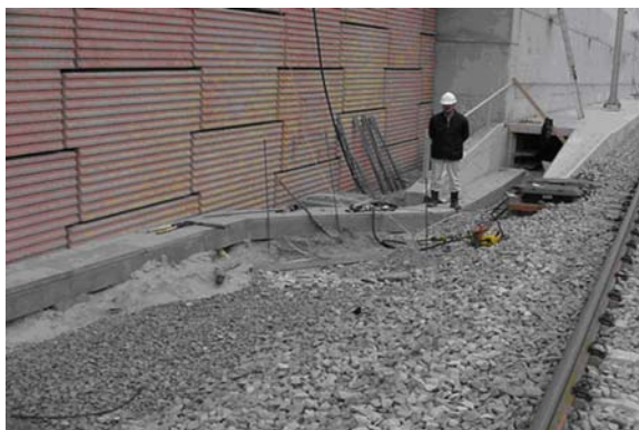
Figure 23. Geomembrane perforation below a underground railway track by installing earth pins for de-electrification [Dutch railway authorities]
