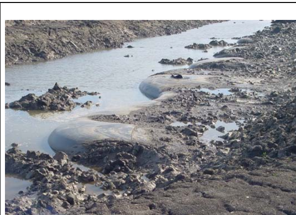
Figure 16. Geomembrane whales due to uplifting water pressure below the geomembrane related to improper backfilling levels [Genap].
