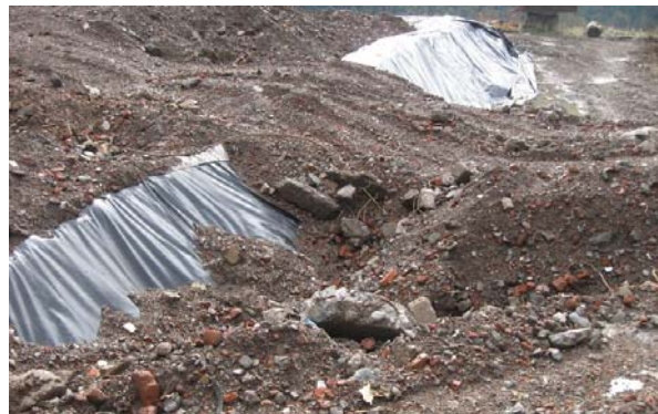
Figure 9. The presence of sharp/big stones without protective geotextiles will significantly increase the risk on damaging the geomembrane [Gerritsen].
