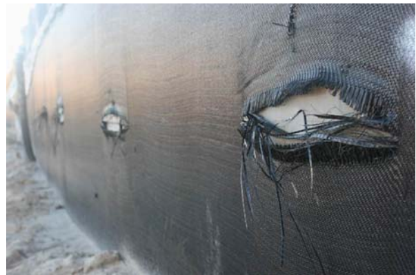
Figure 20. Mechanical damage of a woven protective geotextile by handling of heavy equipment, given a direct threat to the geomembranes behind [Gerritsen]
