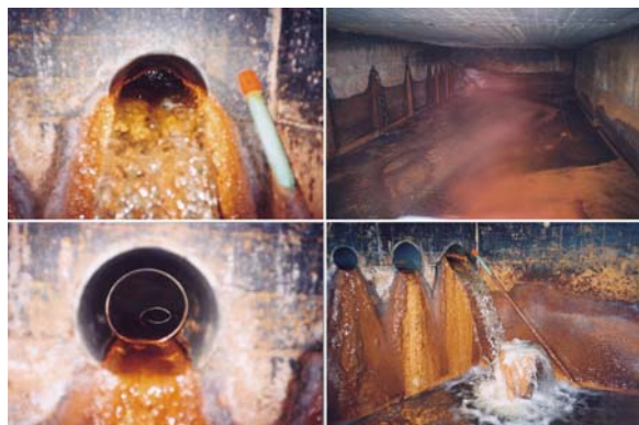
Figure 24. Inspection of a water collection cellar, observations of an increased influx (leakage) with external iron rich groundwater, blocking the total drainage system within a geomembrane construction [Municipality of Zwolle]
