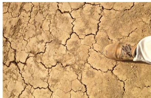
Figure 10. Unacceptable desiccation of clay sub grade [Scheirs]
