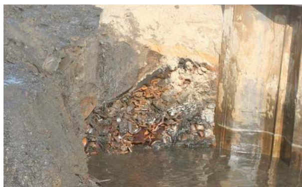
Figure 8. Presence of an un-expected dumpsite with ceramic material and environmental pollutions at a project site with a planned submerged geomembrane [Gerritsen].
