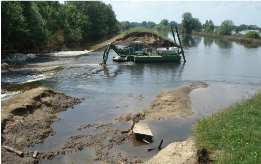
Figure 1: Levee breach in village Račinovci
