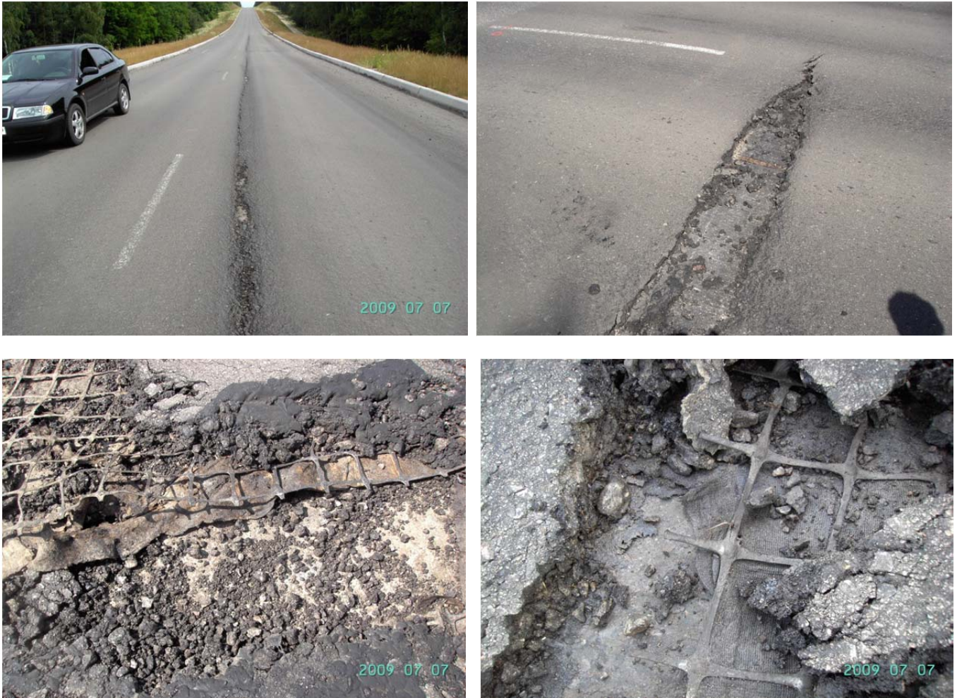
Fig. 2. View of the section on the descent and disruption of asphalt concrete pavement in upper part of section.
