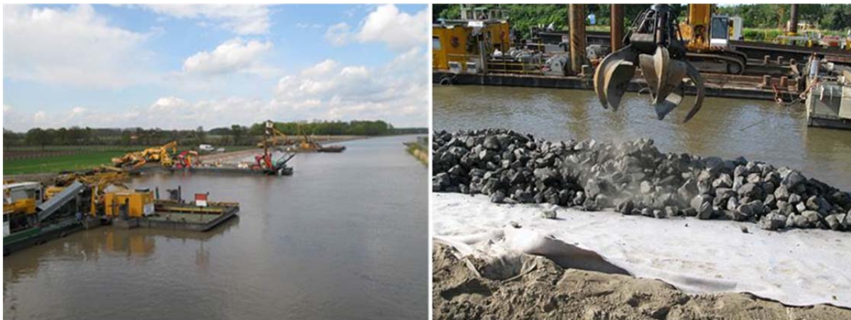
Figure 1: Placement unit for geotextiles and armour stone installation (left) and dropping of armourstones (right)
