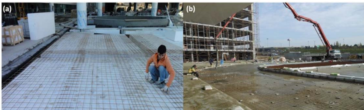
Figure 4: Reinforced concrete load distribution slab construction steps (a) Placement of Q257 / 257 reinforcement, (b) Concrete pouring for driveway
