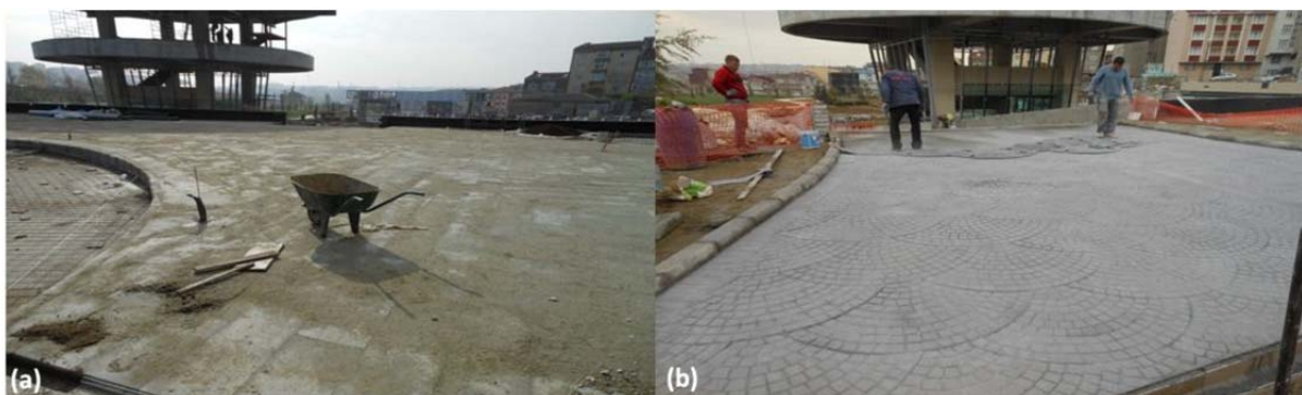
Figure 5: Pavement construction (a) Pavement stone application in sidewalks, (b) Stamped concrete application in driveway
