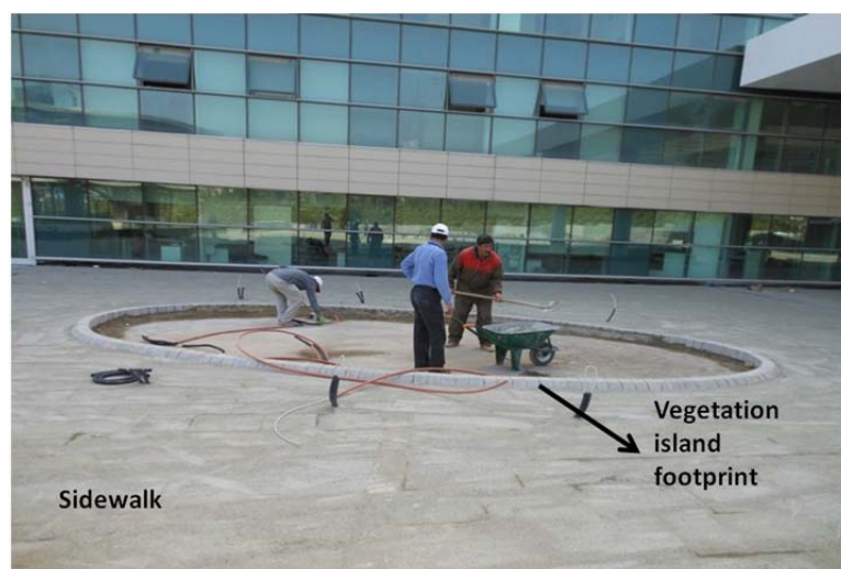
Figure 7: Site preparation to apply geocomposite drainage layer at the footprint of one of the planted recreational areas in sidewalk
