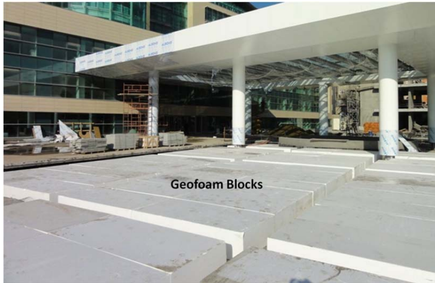
Figure 3: Geofoam block layout over the reinforced concrete slab of existing parking structure
