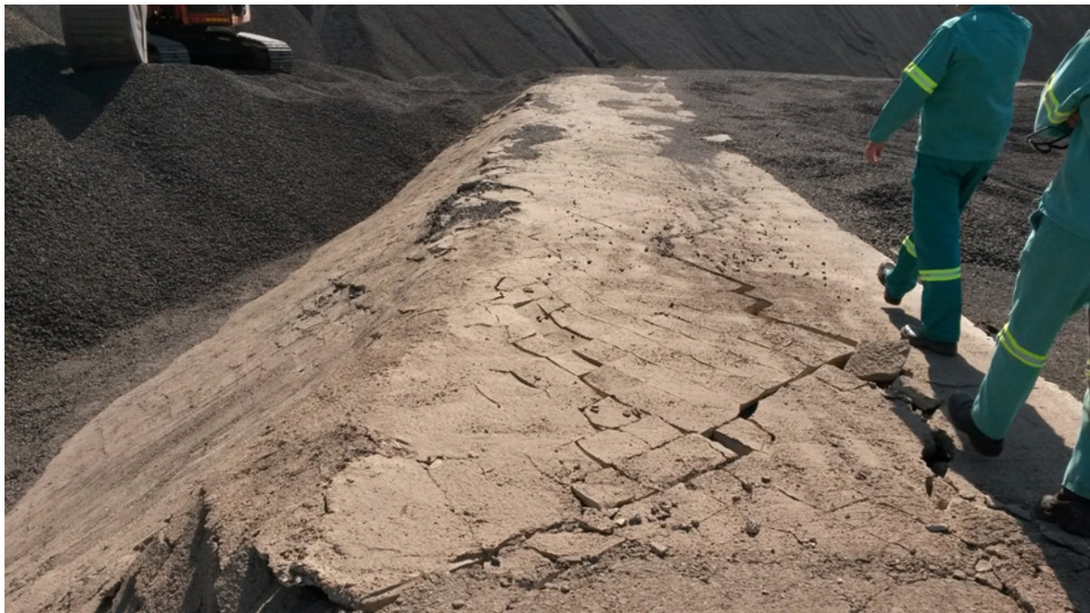
Figure 2. Large cracks in the existing capped side slopes.
