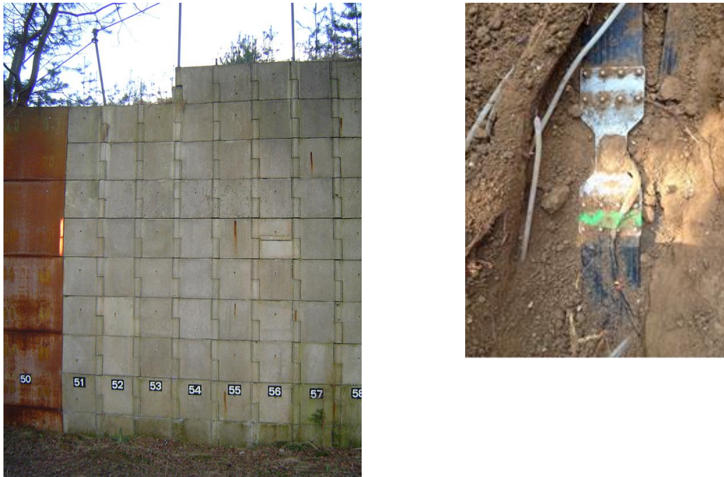
(a) (b) Figure 2: (a) External view of section containing polymeric reinforcement and (b) Exhumed sample from 2014 showing original strain gauge used during TRL monitoring programme
