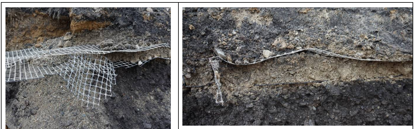
Figure 5. Original reinforcement provided for mining influence at the A4 highway (section Ruda Śląska – Chorzów).
