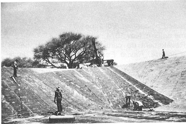
Photo 6. Reservoir lined with Bituminous geomembrane at Goudel, Niger
