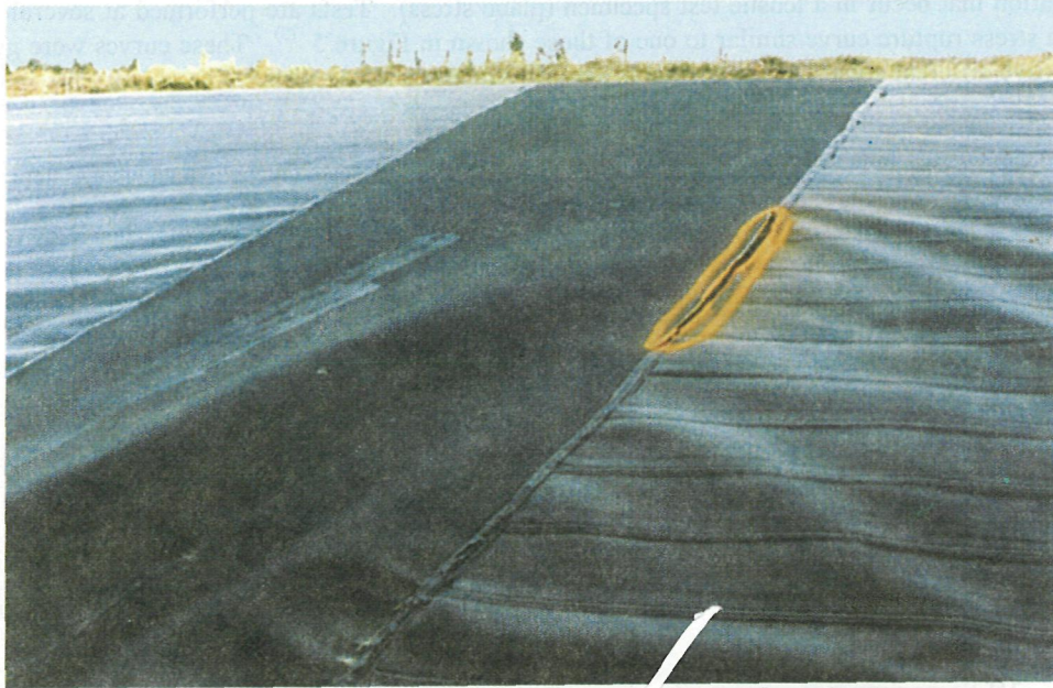
Figure 3 Typical Stress Crack At Edge Of Seam
