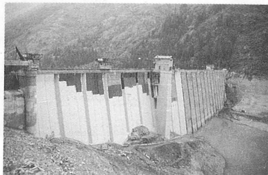
Figure 9. To minimise impact on operation, large panels are prefabricated and installed horizontally, to follow the raising of the reservoir
