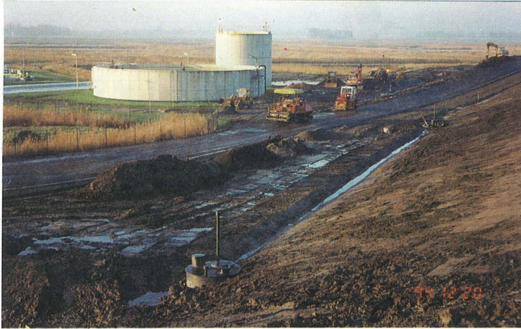
Photo 5 View showing leachate collection control point and treatment plant
