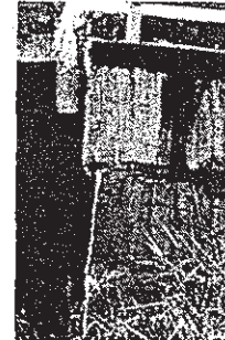
Figure 4. Wall face rotation and damages.
