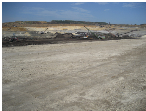
Fig. 7 Excavated slope in the improved soft soil masses, slope inclination 1:6, in the front part uncovered roof of coal layer
