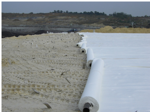
Fig. 5. Installation of geotextile reinforcement on the top of working platform, UTS = 1600 kN/m
