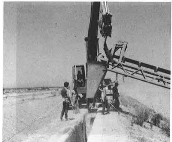
Figure 11: Installation of Center Drain. Geotextile is on Left Side of Trench, Geomembrane on Right Side of Trench.
