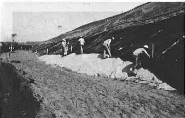
Photograph 4 - Placement of the BD600 over the metabasic soil. During work stoppages the geotextile was protected with opaque plastic covering sheets.
